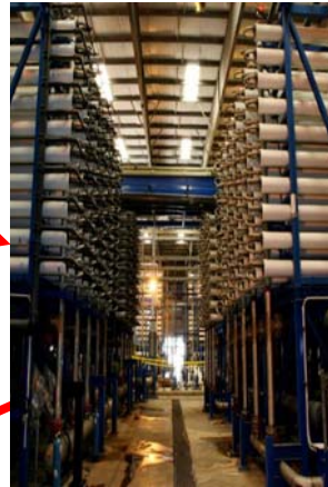
Desalination Plant in Trinidad Tobago
